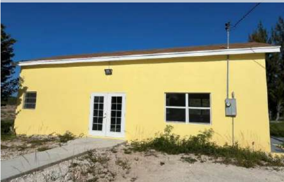
The vegetation growing around the building attracts mosquitoes, which may pose hazards to passengers
