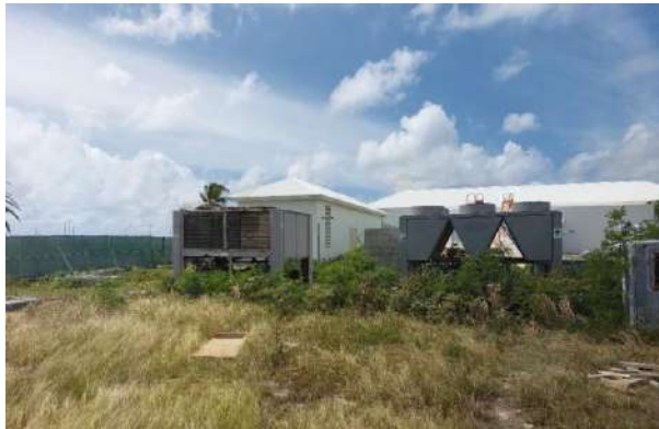
Equipment disposal area, with disabled machinery exposed under the sun, presenting fire risks
