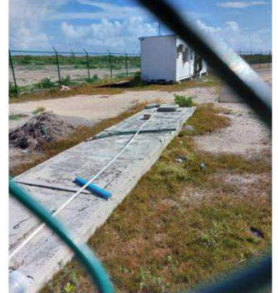
The septic tank and draining system are lacking proper maintenance
