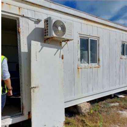
The ARFF facility outworn condition poses a serious environmental and health threat
