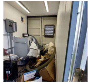
Waste in the generator container creates fire risk and diseases
