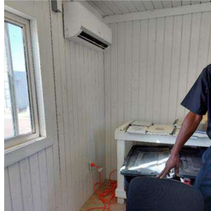
The interior of the ARFF does not have working air conditioning
