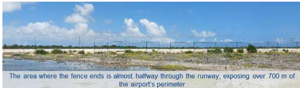
Figure 18. Missing fenced perimeter (expected to be completed by 2024-Q4)
