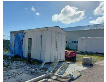
Construction materials laid out throughout several areas, presenting threats to workers
