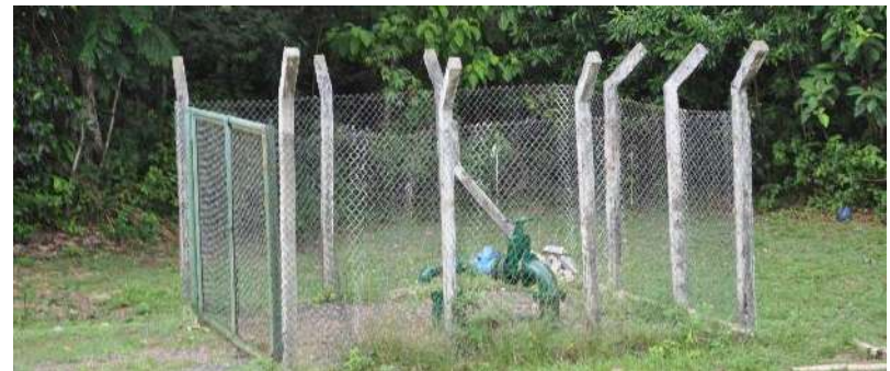
Example: Adequate protection to drinking water in Manaus Airport (Brazil)
